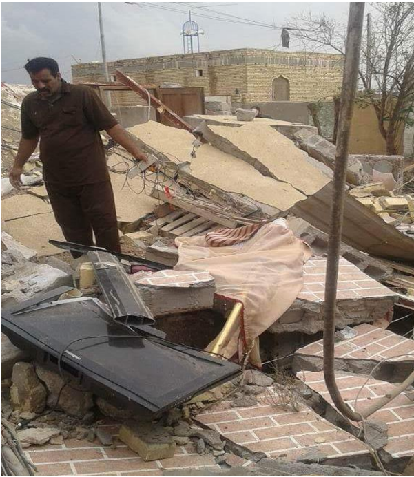
Figure 5. The damage of houses on the path of the tornado
