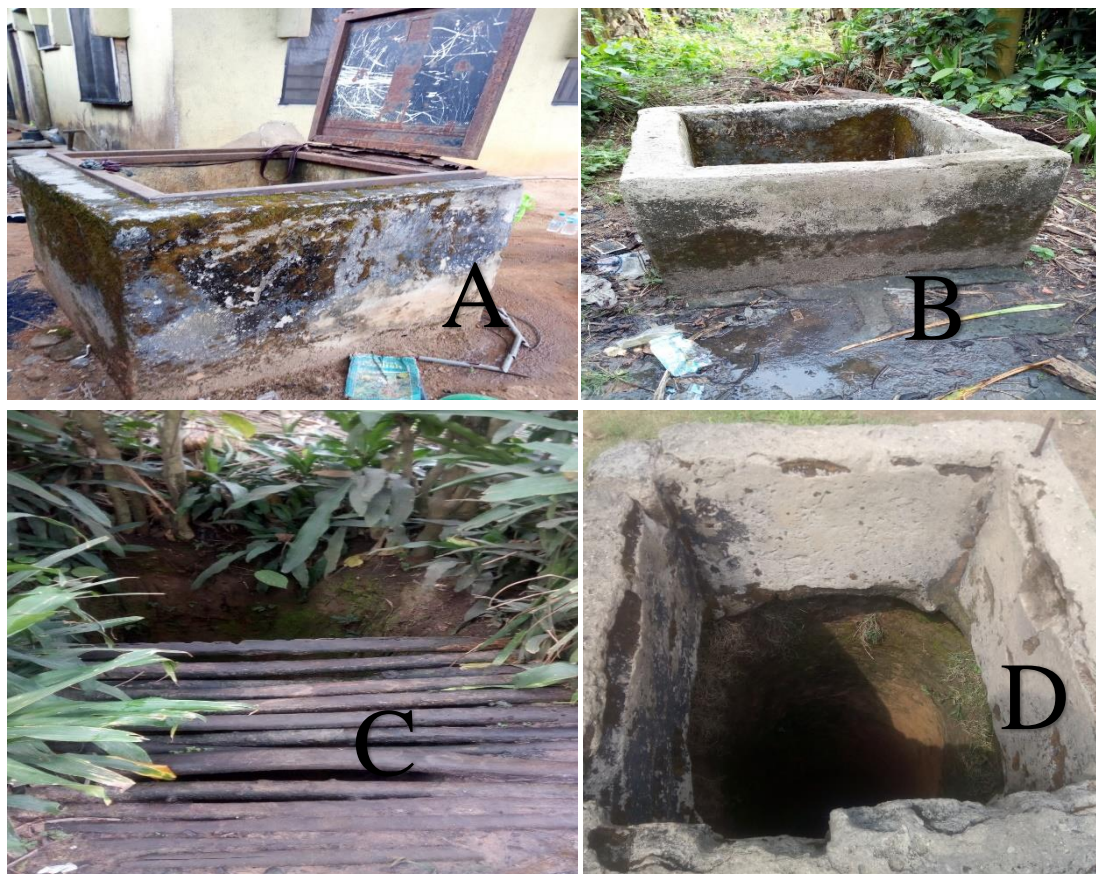
Figure 2. Image of some hand-dug wells utilized as drinking water sources at the sampling stations (A) Eku 1, (B) Samagidi, (C) Eku 2, and (D) Okuechi.
